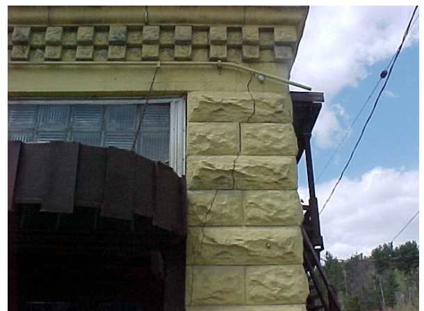
Figure 3 - severe structural damage to a masonry building in Ausable Forks, NY
